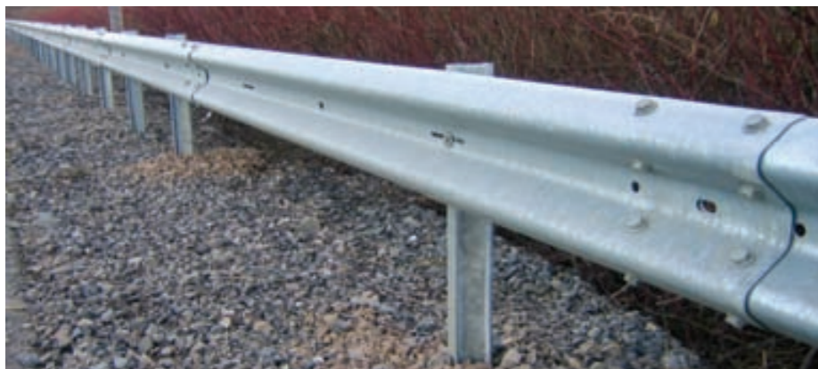
Normal containment barrier
