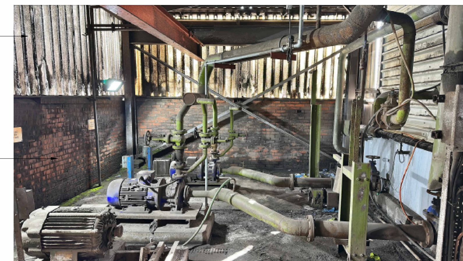
Photo 3 - RH Pump House
