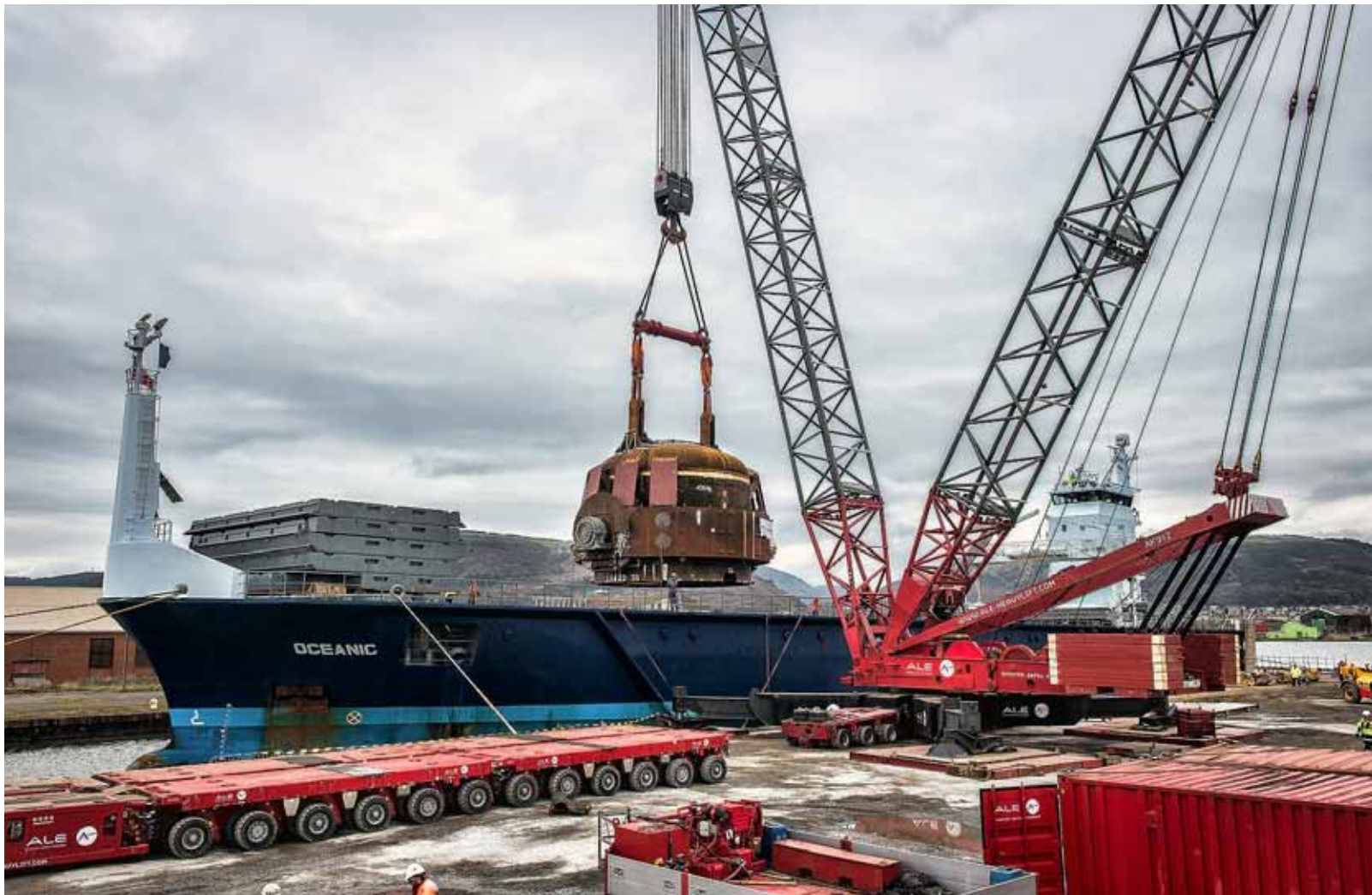
The 450-tonne converter shell was lifted out of 'Oceanic' onto a low-loader and driven carefully on site
