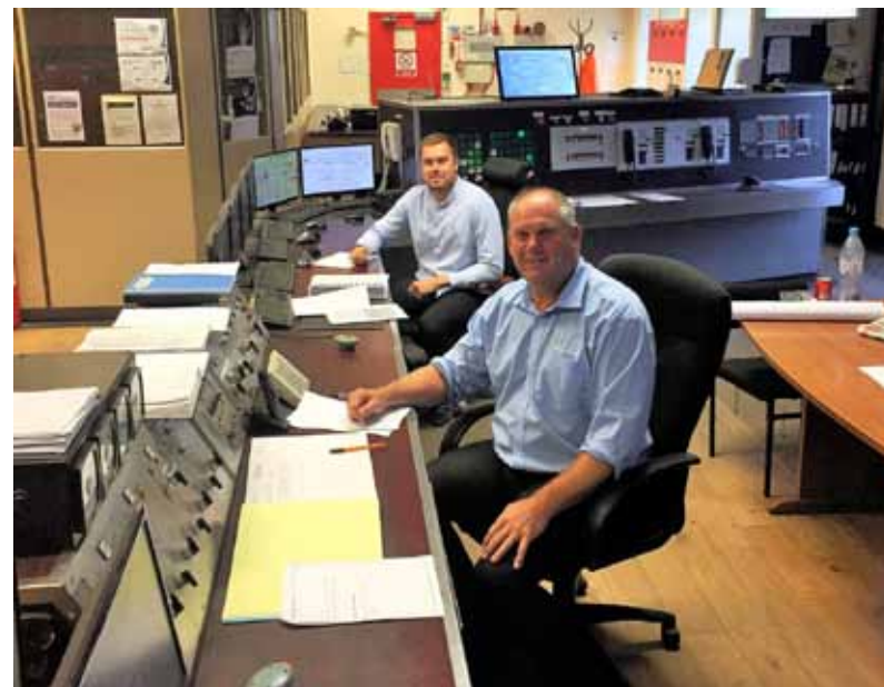
Scott and Phil, keeping a watchful eye out at Port Talbot's Energy Control
